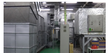
Revamped exhaust gas treatment system for the removal of THF
