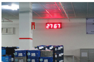
The temperature and humidity indicator panel that has been installed
